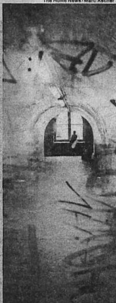
The pedestrian tunnel under the tracks as seen through a graffiti-covered window. The smell in the tunnel is a frequent focus of complaints.
