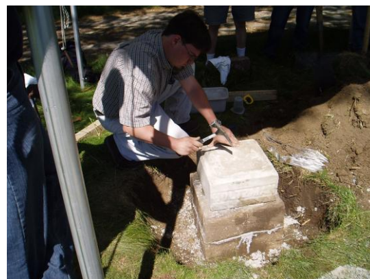
Treatment: Typical resetting/leveling of base (not this site – NCPTT Cemetery Conservation Workshop 2005).
