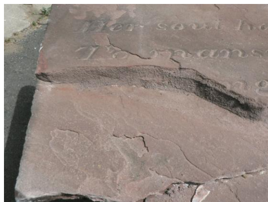
Treatment: Typical patching for delaminated boundary (not this site – First Presbyterian Church of Elizabeth, NJ, 2007).
