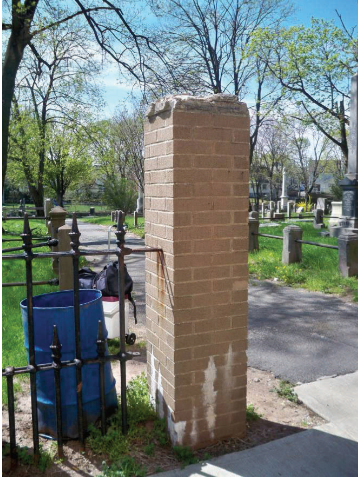
Photo 32: A typical masonry pier. These date to the late twentieth century and are currently in poor condition. They do not match the historic gate posts.
